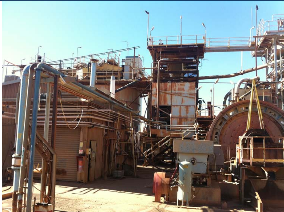
Figure 2: CTP Plant under consideration for refurbishment
